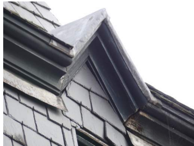
Afb. §24.04, detail gescheurde, ingewaterde verbinding
