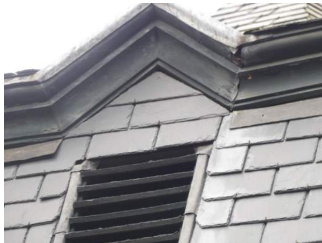
Afb. §24.03, detail gescheurde, ingewaterde verbinding
