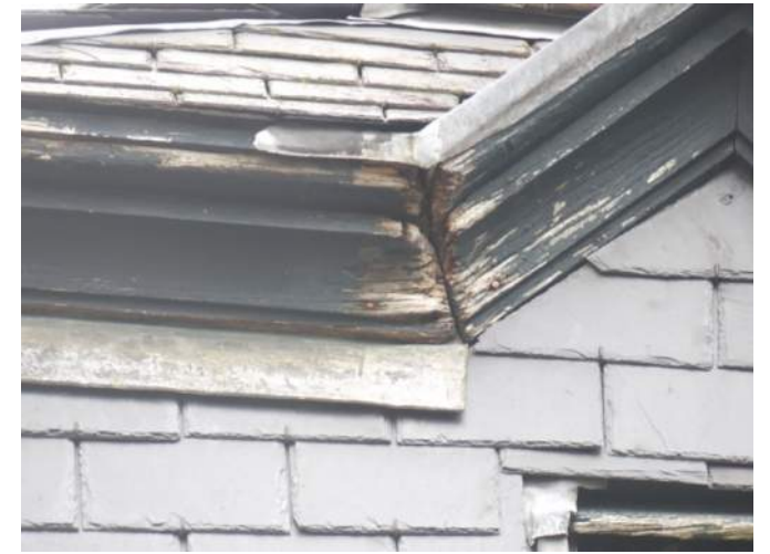
Afb. §24.08, detail ingewaterde, opengescheurde verbinding
