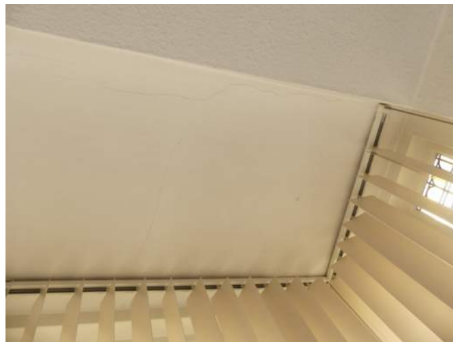
Afb. §40.52, scheuren in erkerplafond
