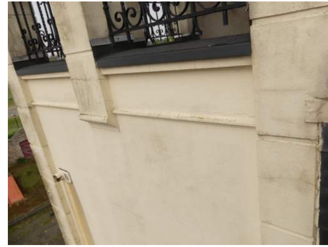
Afb. §40.19, scheuren in torengelvels
