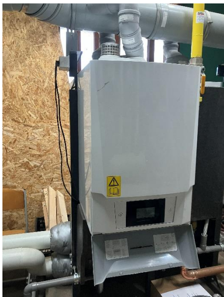
Picture 13: CV installatie
