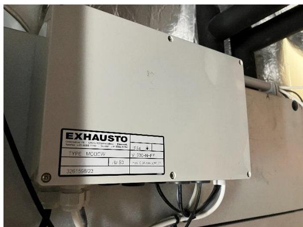
Picture 11: Controller luchtbehandel systeem
