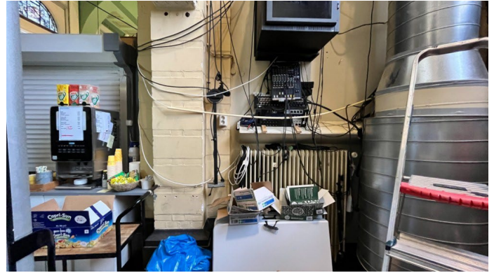
Kitchen of the lunchroom - substandard electrical connections; see risk improvement
