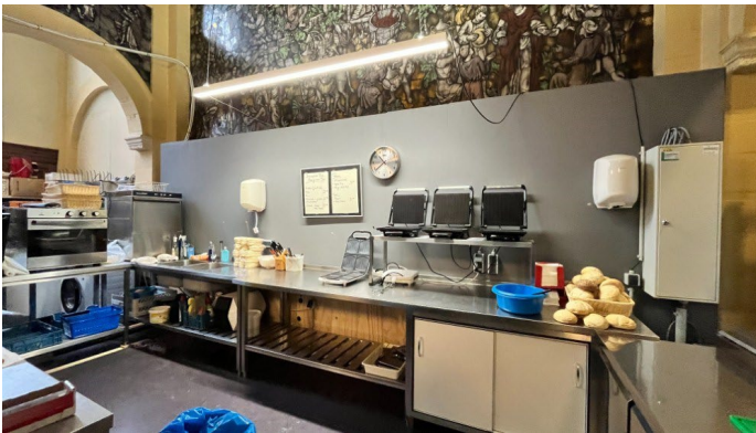
Kitchen of the lunchroom - substandard electrical connections; see risk improvement
