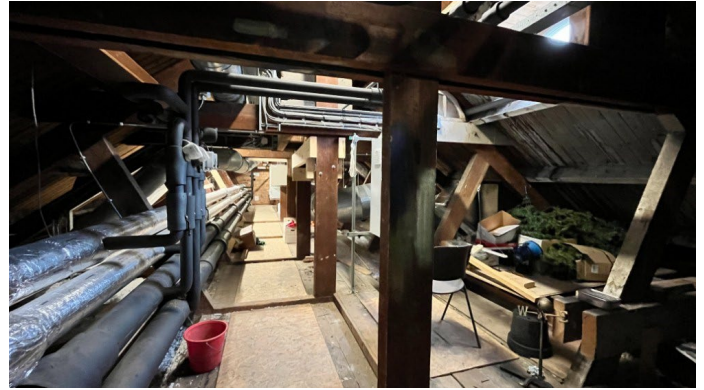
Attic - technical systems and some storage
