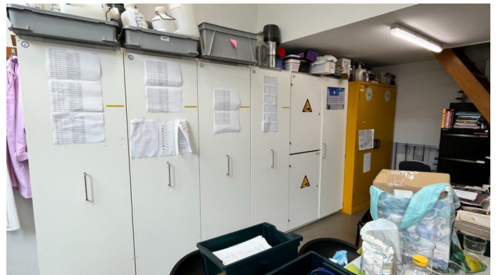
Flammable liquids stored in an approved 30' safety cabinet (yellow) with mechanical extract ventilation
