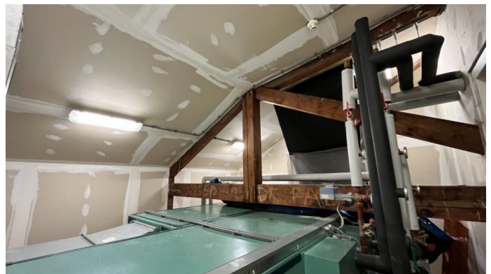
HVAC room; smoke detection fitted here
