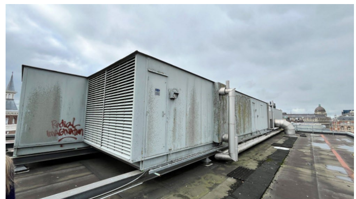
Technical plant room on top of roof, building No 31
