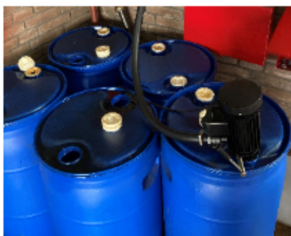
Diesel fuel storage in sprinkler room larger than required
