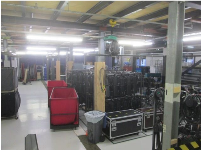
Storage facility under the stage is sprinkler protected.
