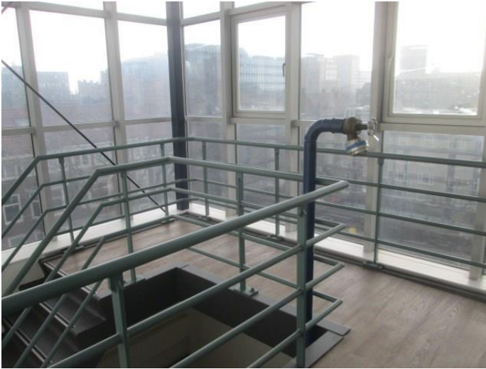
Dry risers in the stairs
