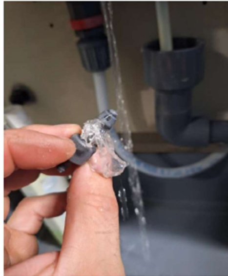
2026 - DR1 - Sample taking unit defect.
