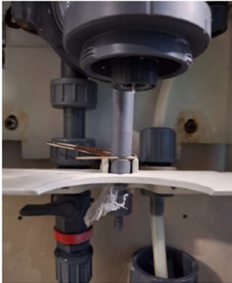
2026 - DR1 - Sample taking unit defect.
