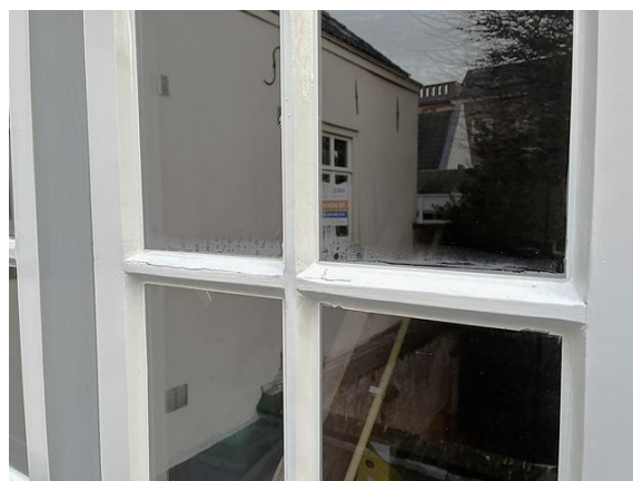
dakkapel no. 6: stopverf losgescheurd (2025)
