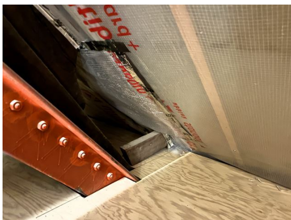
zolder, dak no. 20: blokkeel los (2025)
