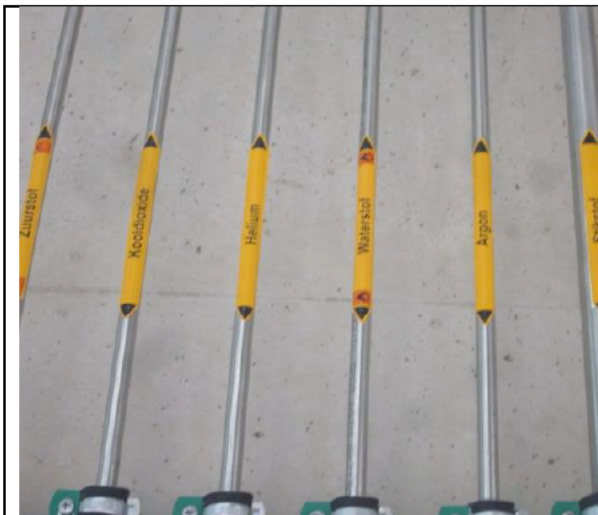
Different kinds of gases with central and decentral valves
