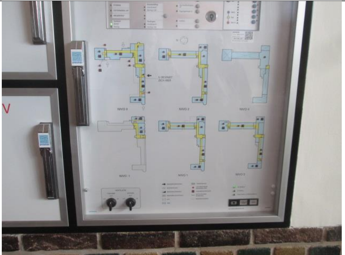
Fire detection panel.
