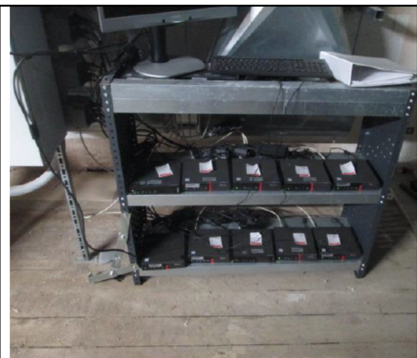
Server like equipment at the attic (see rec.)
