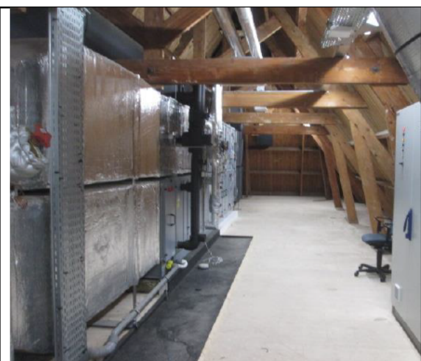
Air treatment system in the attic
