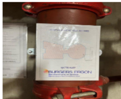
Riser with protection area
