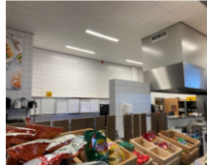
Restaurant - deepfat fryer (R4)
