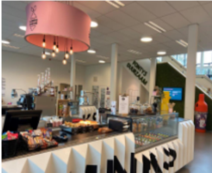
Cafe - electrical equipment (R3)
