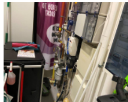
Storage in technical room P7
