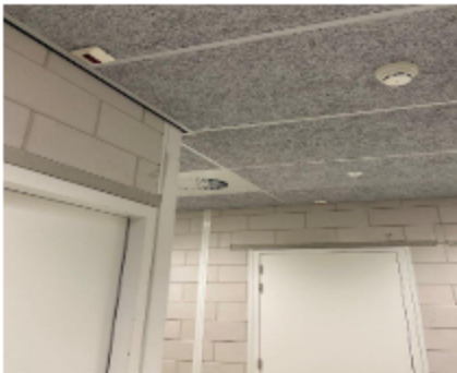
Spot smoke detector
