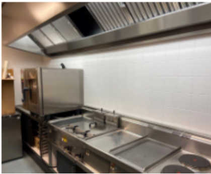
Example of kitchen equipment (in building P4 taken out of order)
