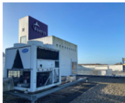
Example roof equipment
