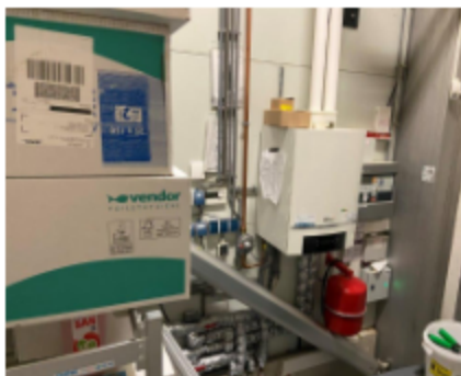
Storage in technical room P7
