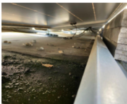
Underneath PV (solar) panel
