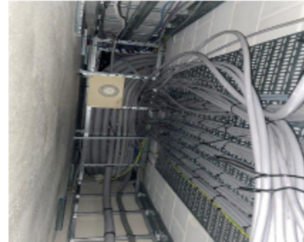
Detection in utility shaft
