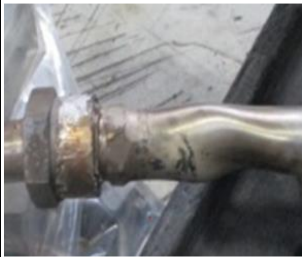
Damaged Water Manifold
