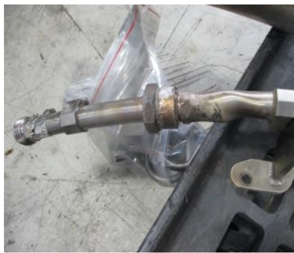
Damaged Water Manifold
