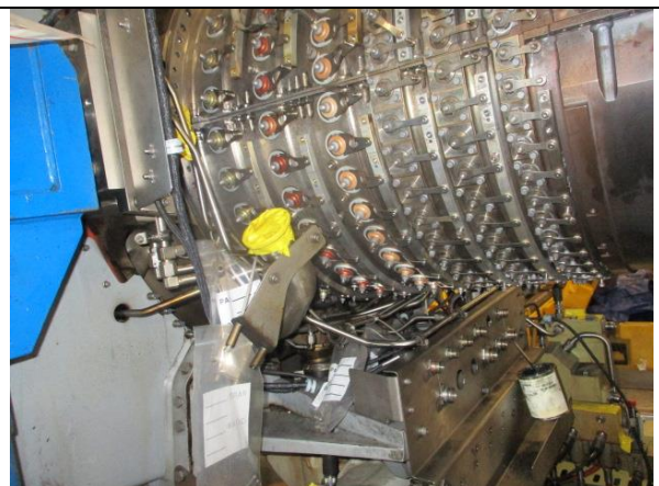
HPC cases installed
