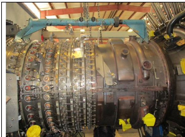
HPC cases installed
