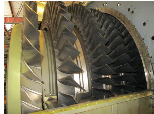
LPC rotor where dry ice cleaned
