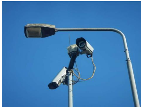
Closed Circuit TeleVision installatie (CCTV installatie), -,
