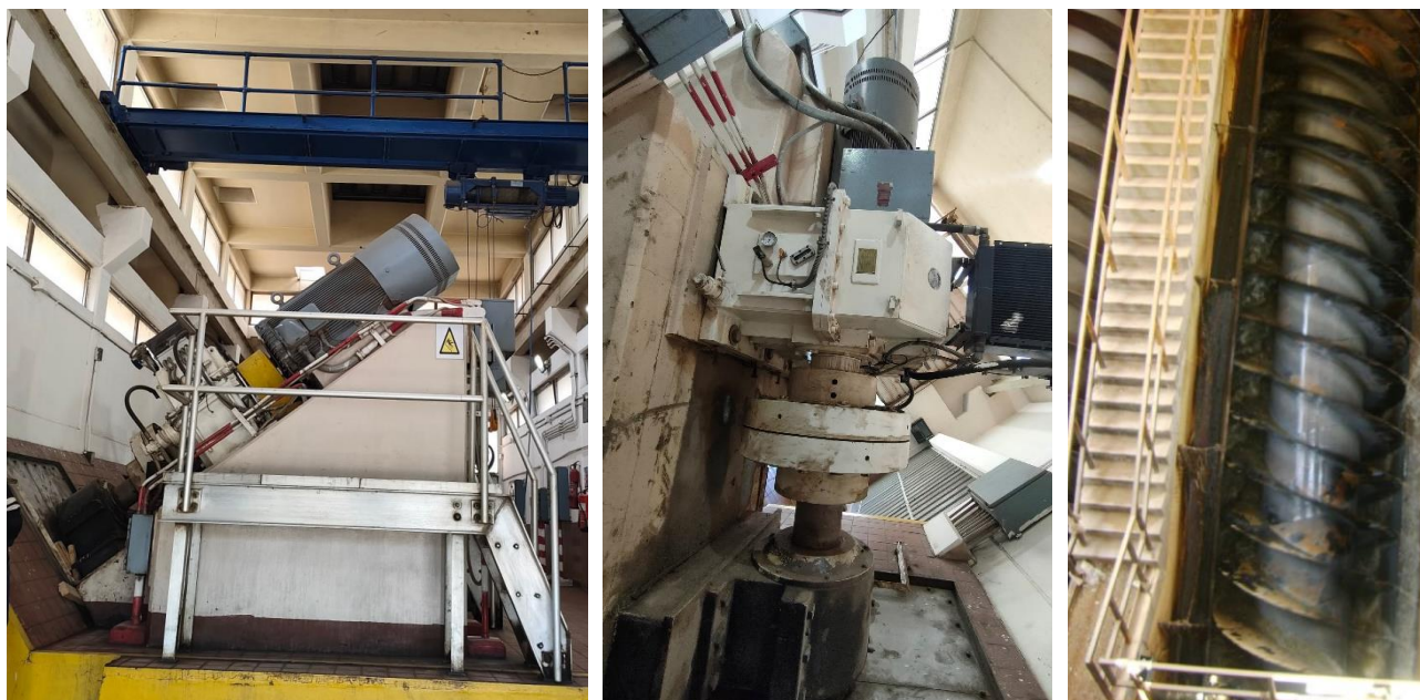
Figure 4. Zenein Pumping Station Complex
