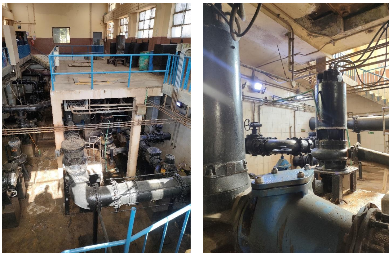
Figure 11. RAS/WAS pump station
