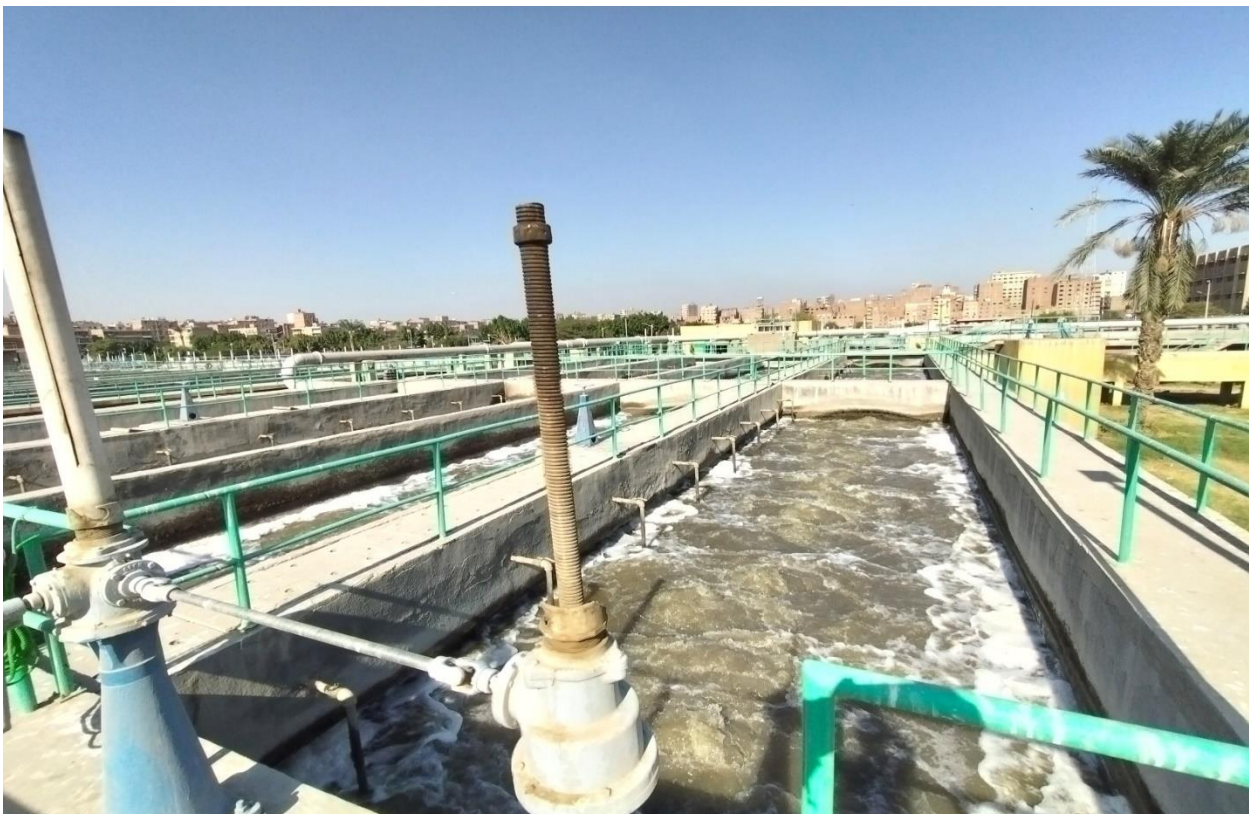
Figure 7. preliminary aeration tank
