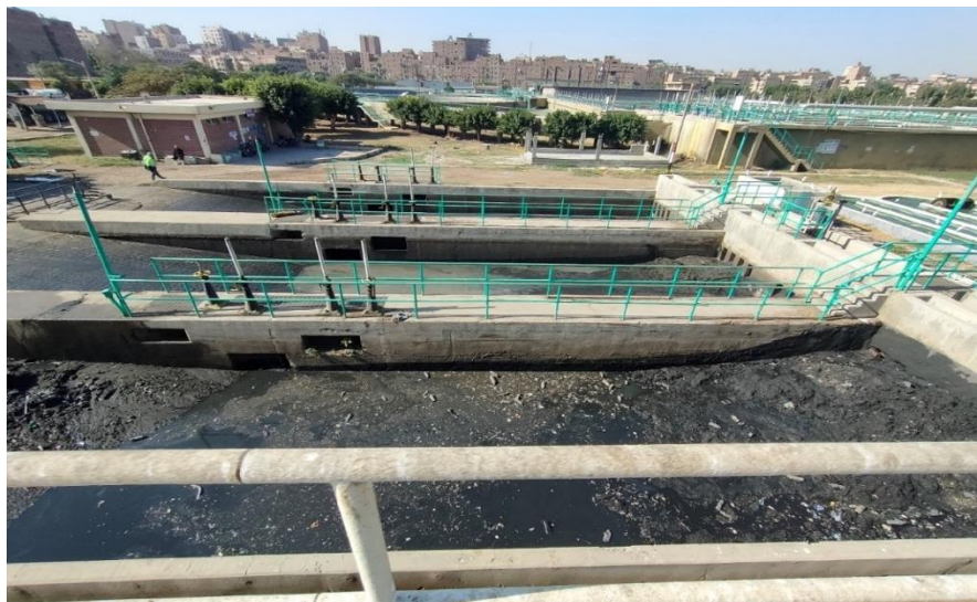
Grit Separation Tanks
