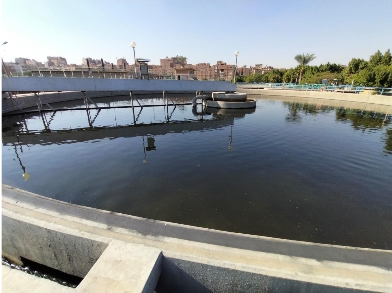
Figure 10. Final Sedimentation Tanks
