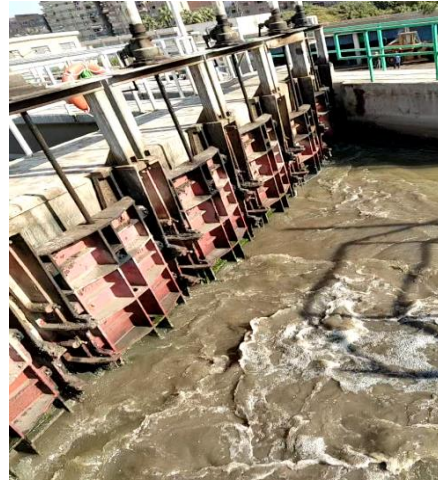
Penstocks at the Grit chambers inlet
