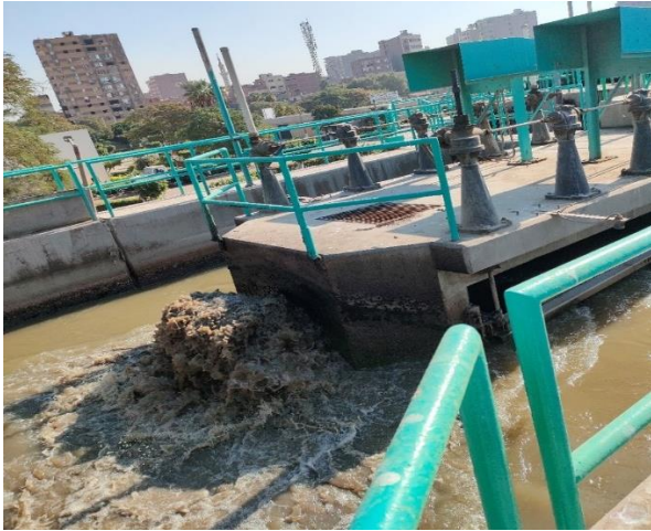
Return Activated Sludge the Headworks
