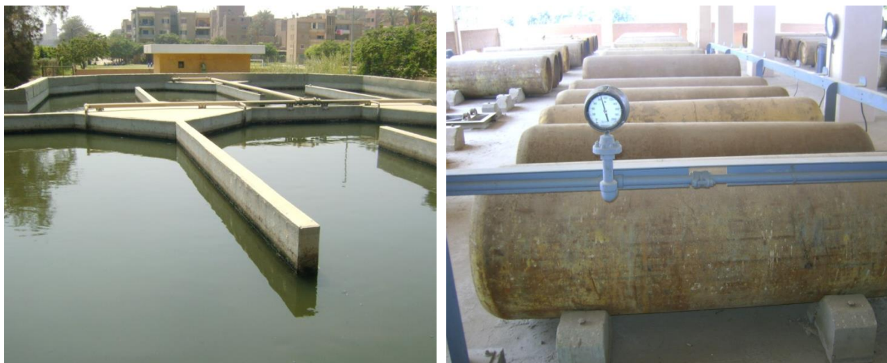
Figure 12. Chlorine Contact Tank
