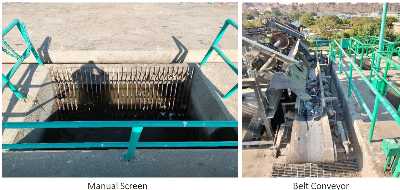
Figure 5. Mechanical and Manual Screens
