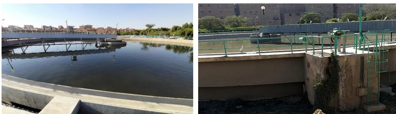
Figure 8. Primary Sedimentation Tanks
