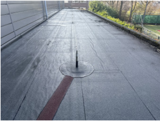
Lage dak links achter
