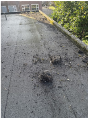
Lage dak links achter vuil
