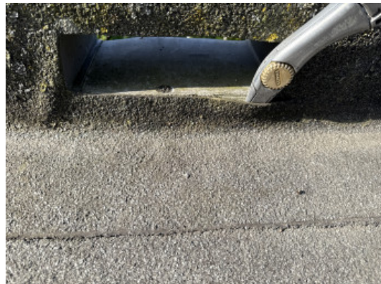
Lage dak links achter noodoverstort lek
