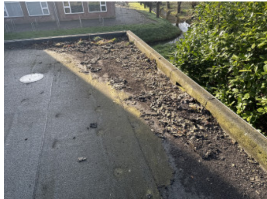
Lage dak links achter vuil
