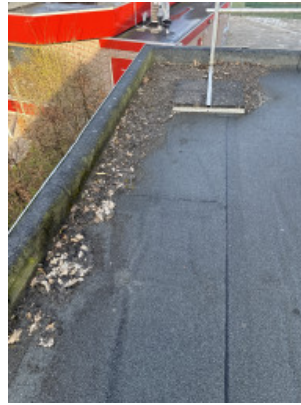
Lage dak links achter vuil
