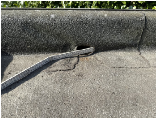
Lage dak links achter hwa lek
