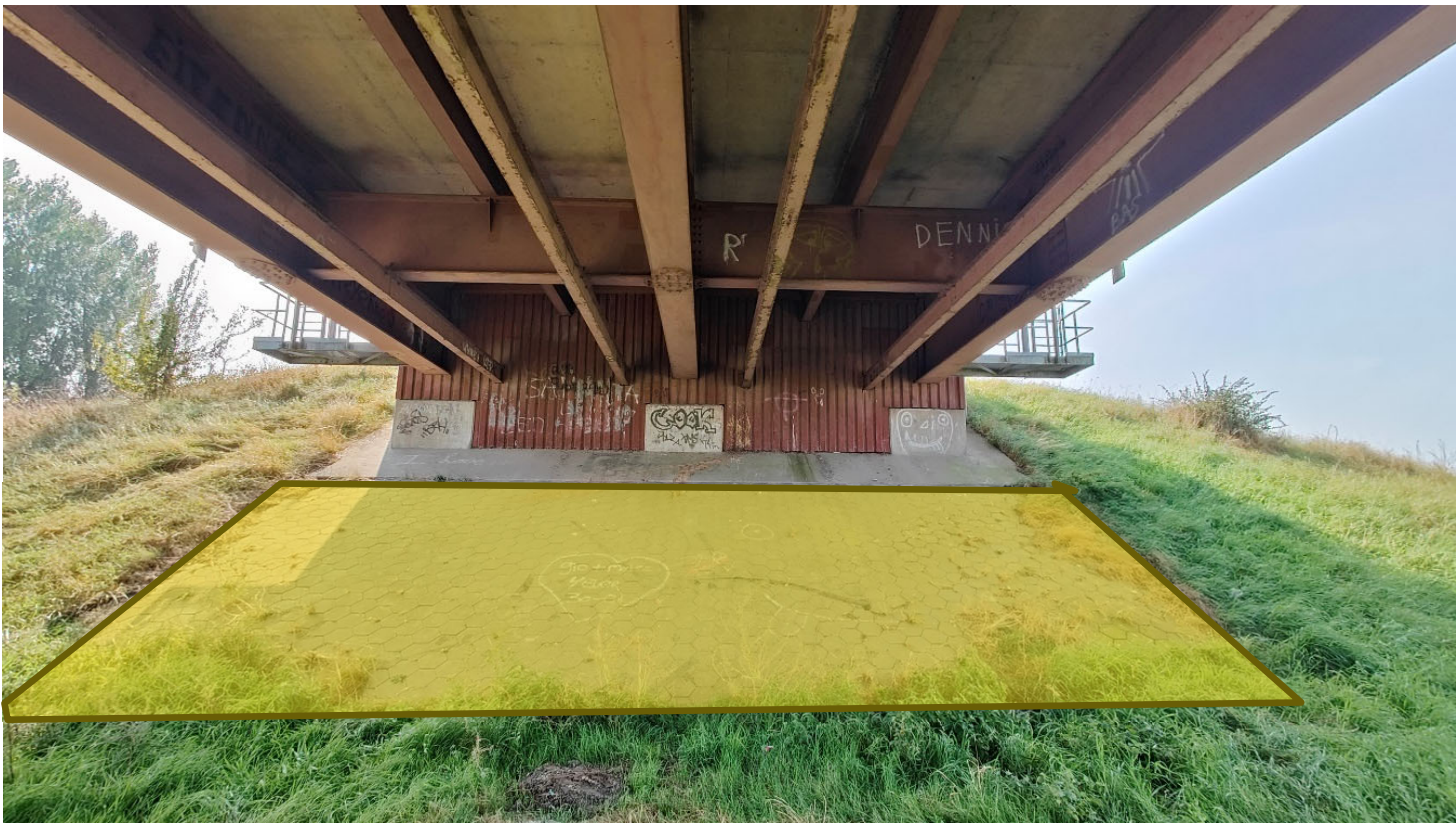
STP 01 (LH WEST)
