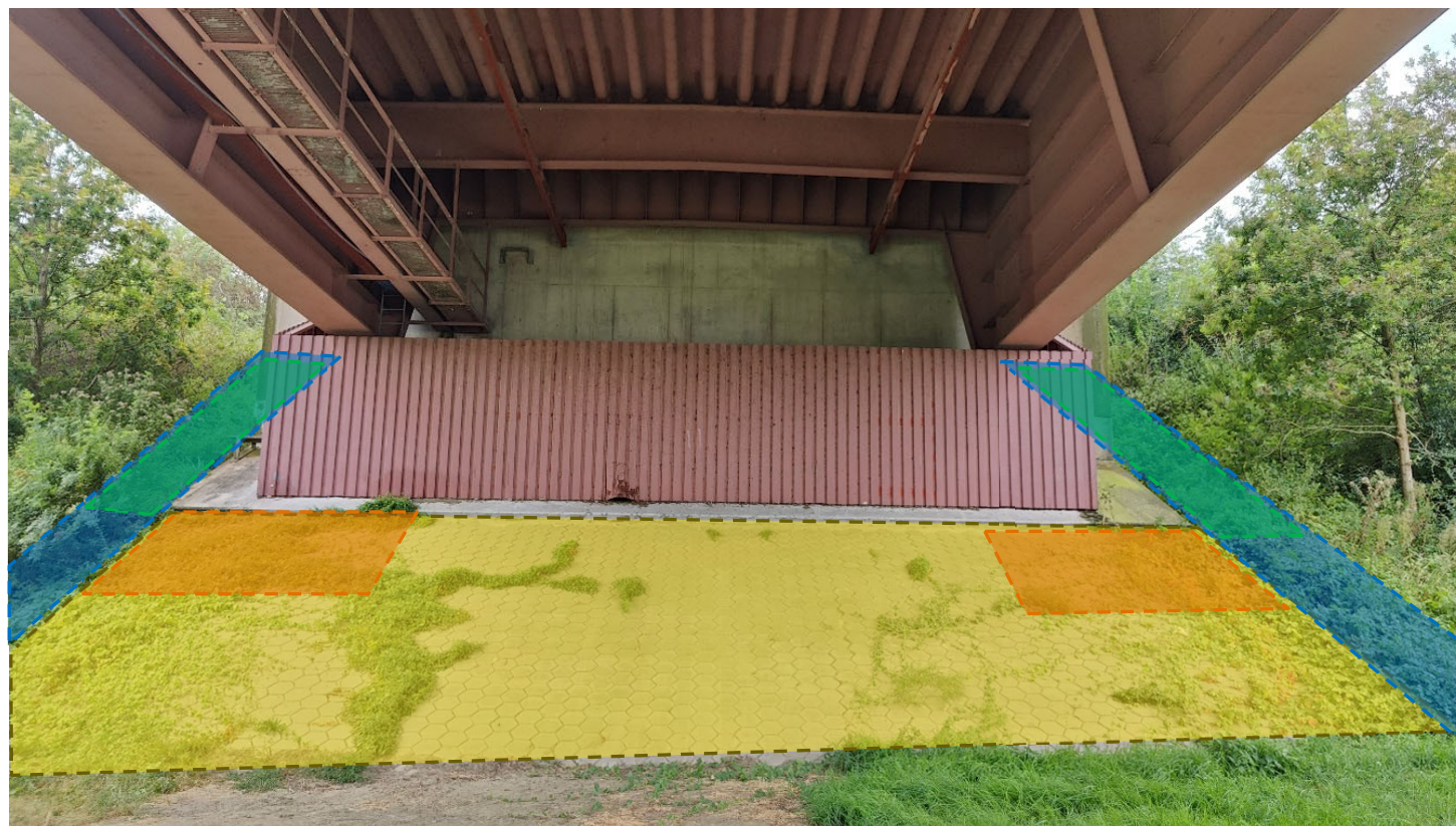
STP 01 (LH WEST)
