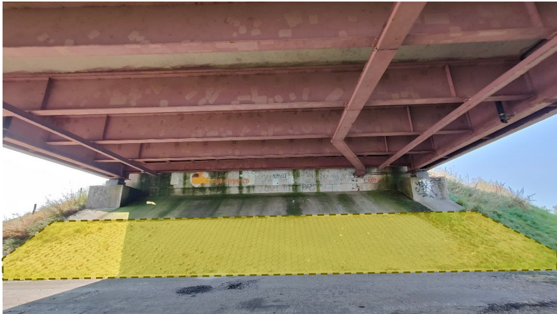
STP 04 (LH WEST)
