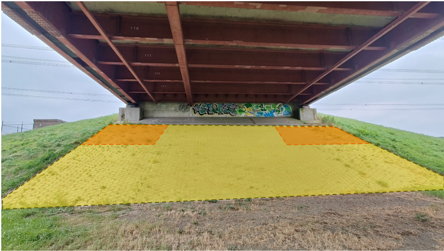
STP 01 (LH WEST)
