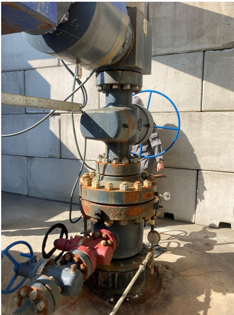
Figure 17 Wellhead of MDM-GT-03-S2 (in operational setting).
