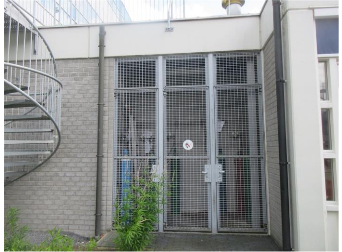
Storage of inert gases
