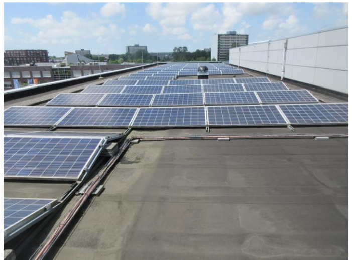
Solar panels, mineral insulation roof
