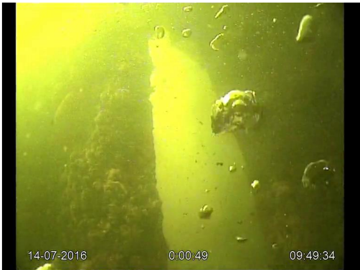
Gat in damwand 4mtrx 50cm.
