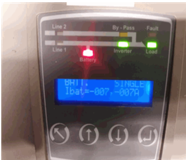
UPS on battery
