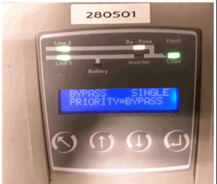
UPS in interne bypass
