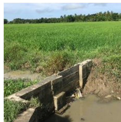
Figure 96: Example of a sluice in the Ayeyarwady Delta
