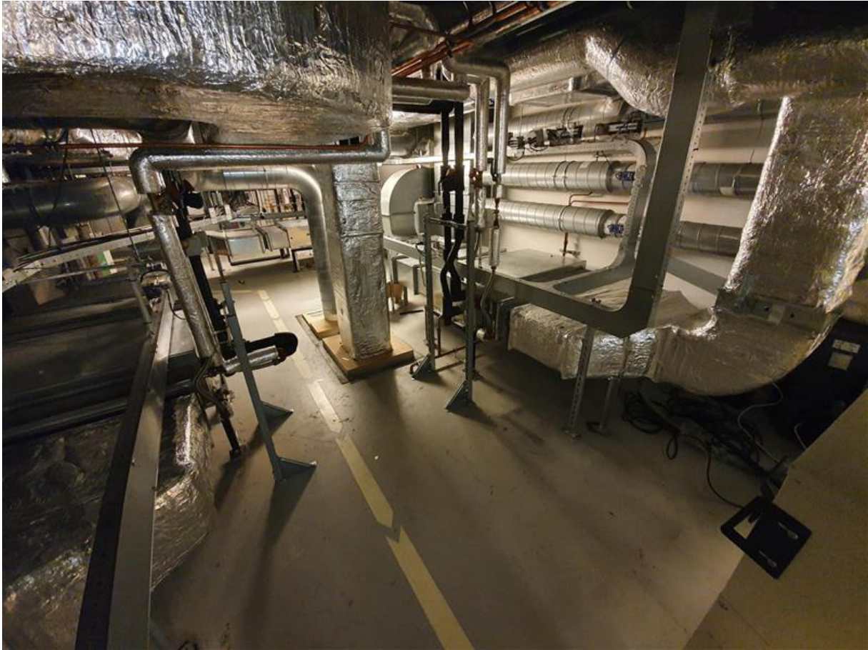
Figure 6: Photo taken in the technical room on opposite side of figure 5, from top left position in figure 3; Space available for placement of the GHS depicted by area (A) and area (B). Area (C) which requires periodical access resides between the wall and the cable tray.
