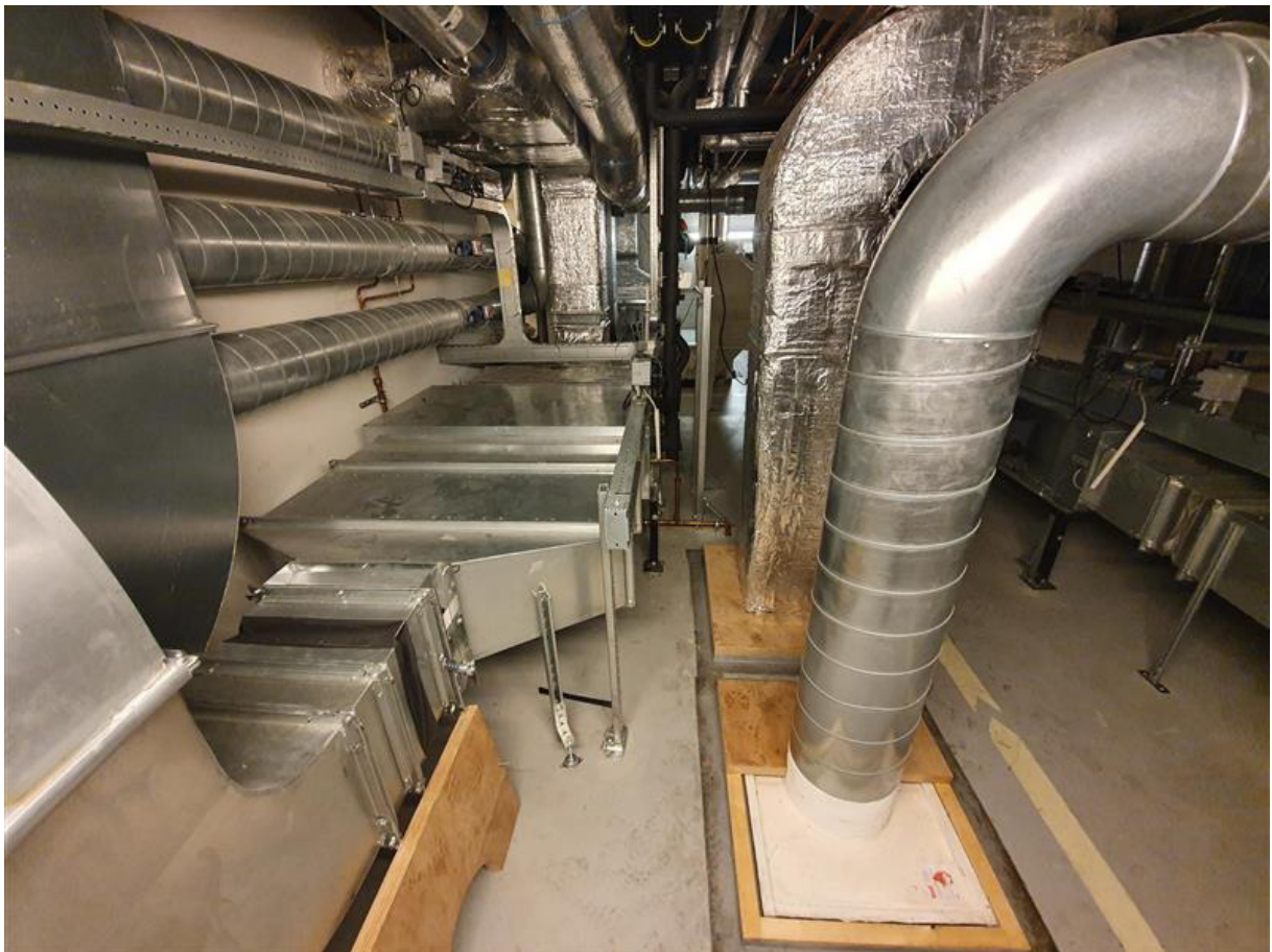
Figure 5: Photo taken in the technical room from right upper corner in Fig. 3; white area in the bottom right of this photo is the feedthrough with air conditioning vent ((D) in Fig. 3) that can be used to pass the lines between the cryostat and peripherals placed in the technical room. The photo also shows a clear LOS towards the intended GHS position.
