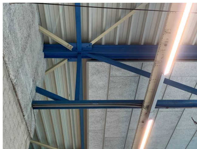
Corrosievorming vakwerkspant as 27
