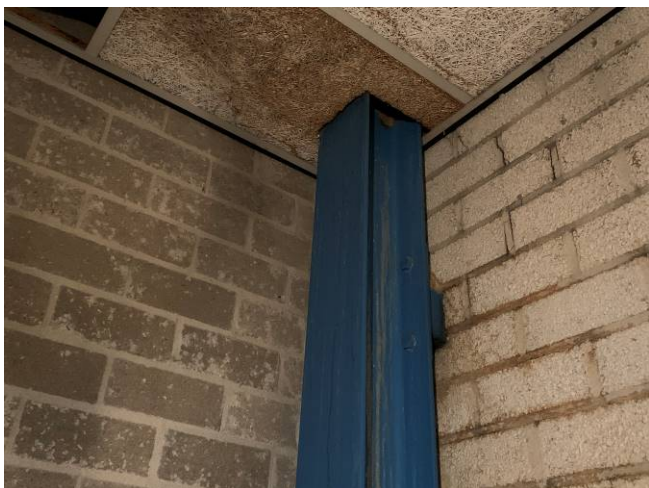
Lichte corrosievorming kolom as C28
