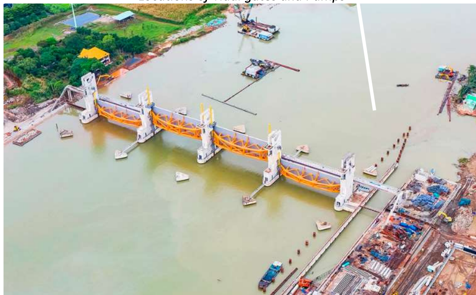
Tidal gates at Muong Chuoi location (4x40m and lock)
