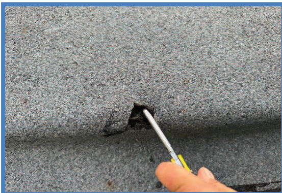
Scheur in dakbedekking
