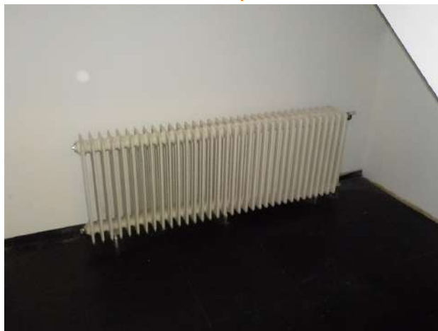
Radiator in trappenhuis begane grond
