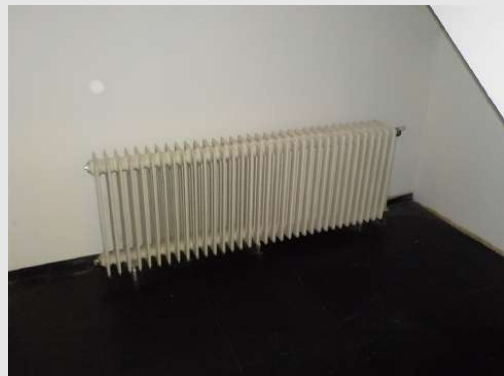
Radiator in trappenhuis begane grond
