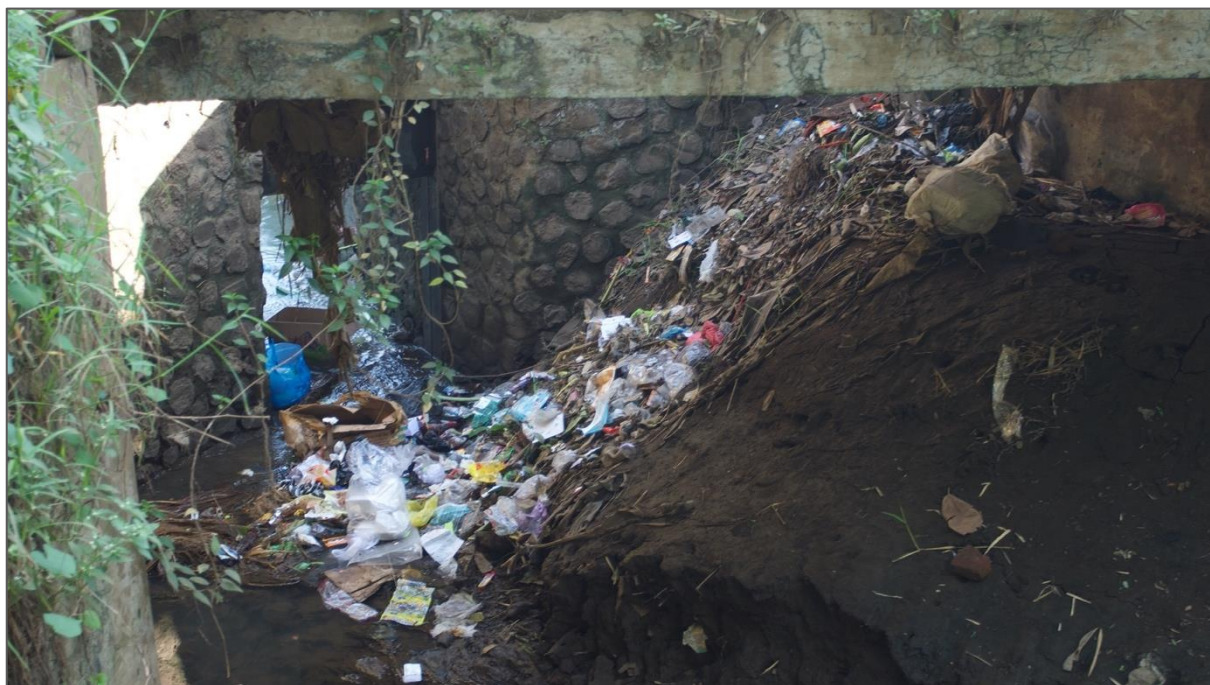
Figure 5.13. Solid waste accumulates in channels and drains.
