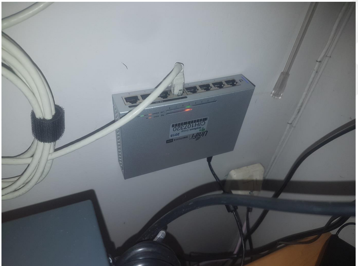
Switch in kantoor
