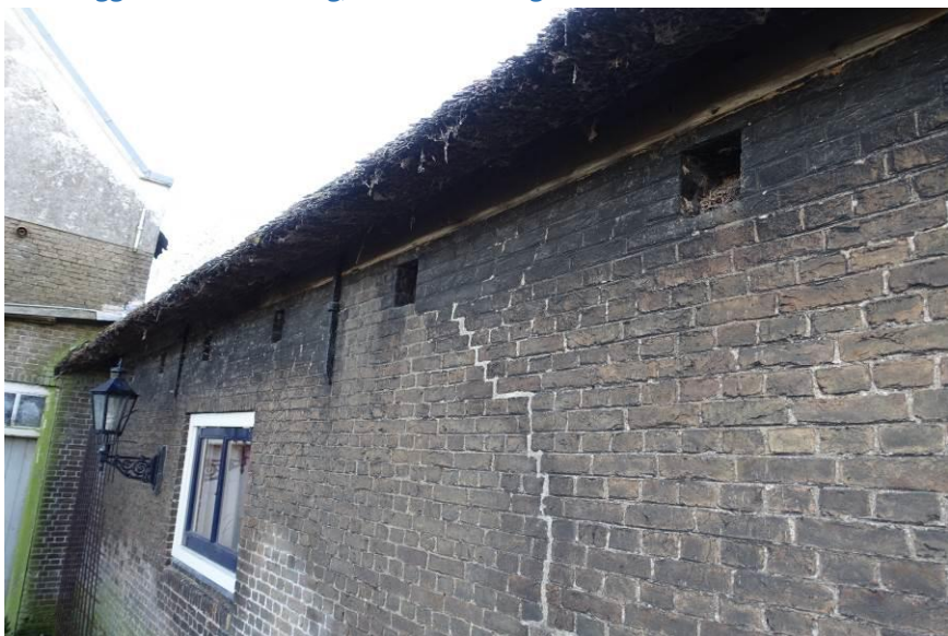
Scheurvorming in gevels.
