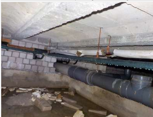
De riolering is van pvc
