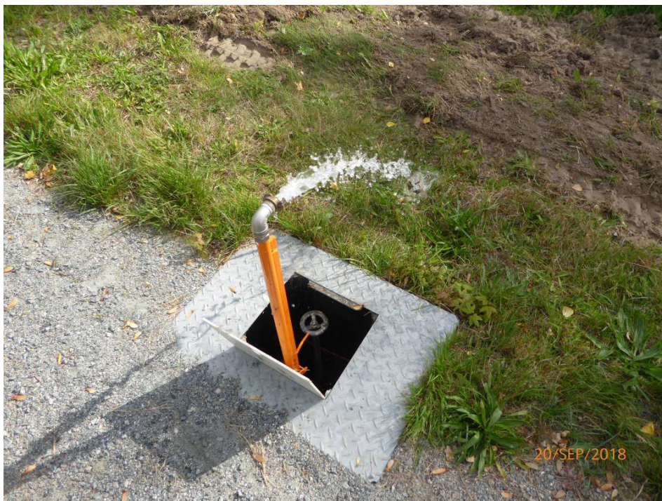
Figuur 25 Hydrant/Was & vulhydrant B2
