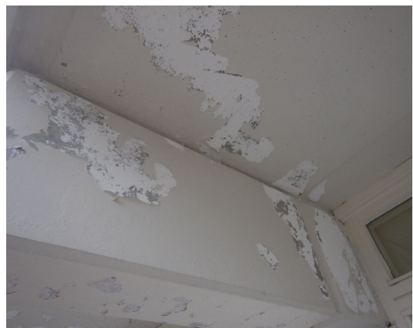
Figuur 6.17: Schade coating console
