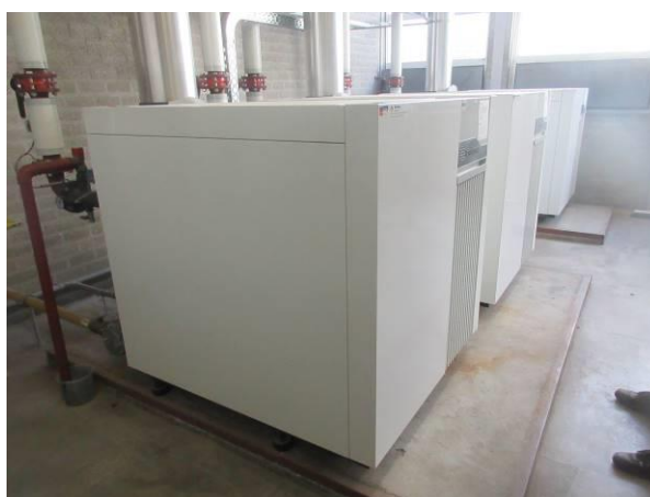
CV-ketels in ketelhuis
