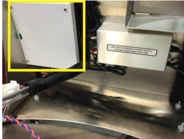
Figure 14 - Back Control Panel
