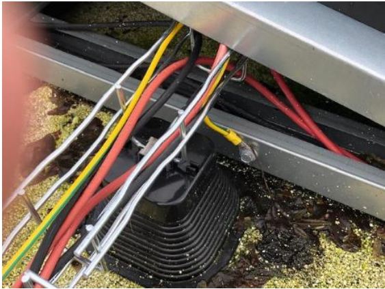
Bedrading in open goten
