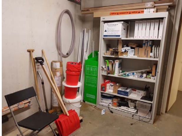
Housekeeping Sprinkler Room
