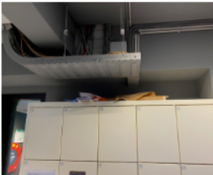
Storage close over electrical cabinets
