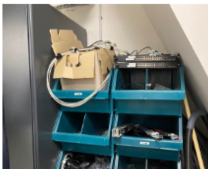
Technical room storage
