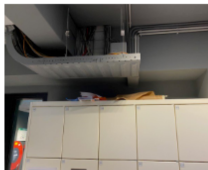
Storage over electrical cabinet
