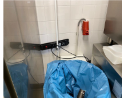
Storage in Electrical room
