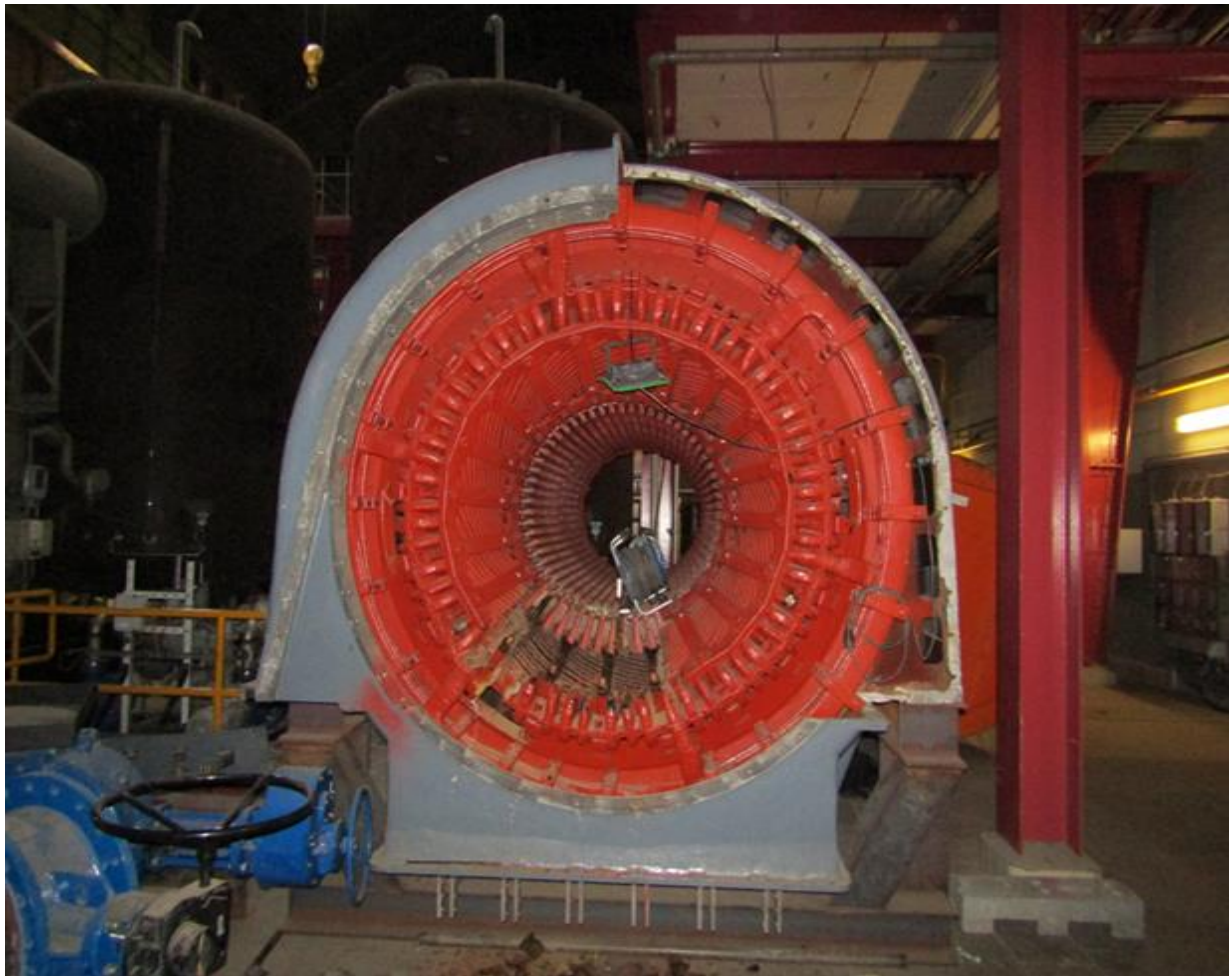
Connection end (CE) spare stator
