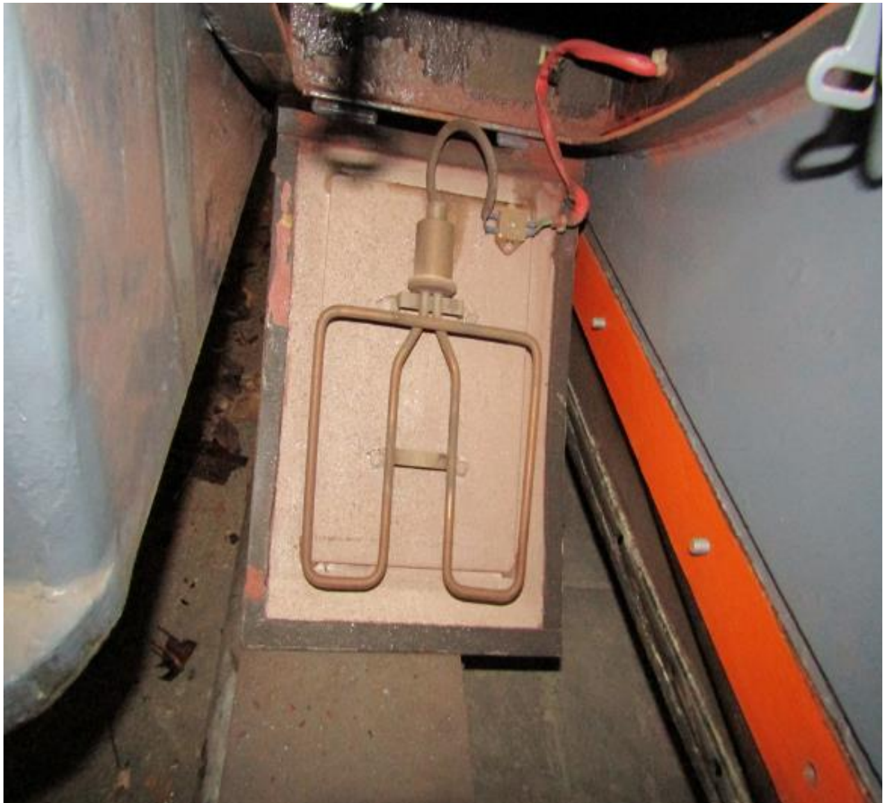
One of four spaceheater
