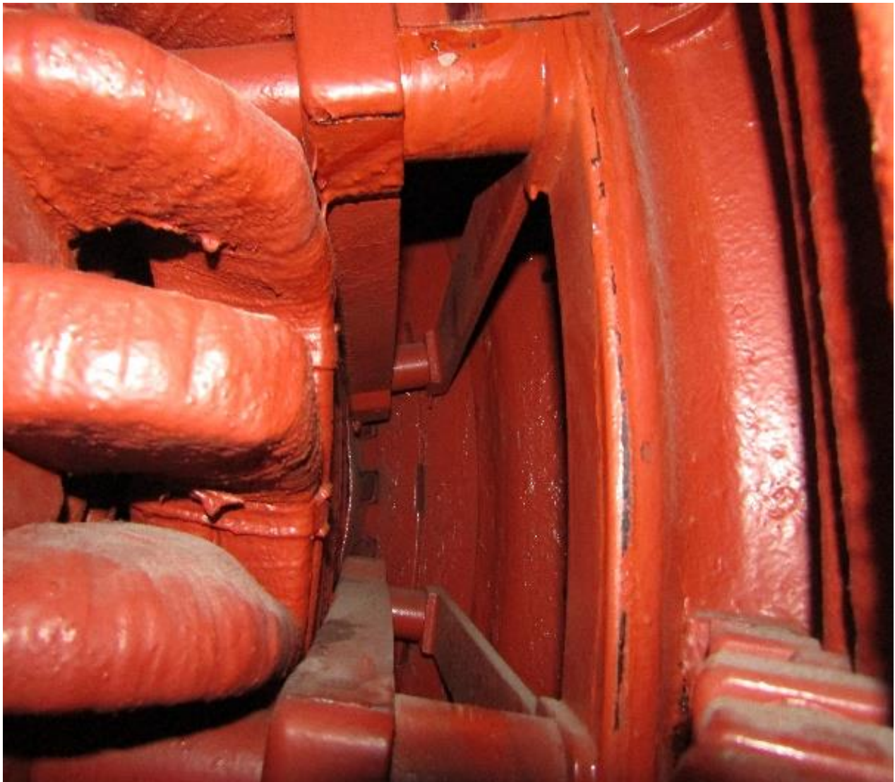
Windinghead support system
