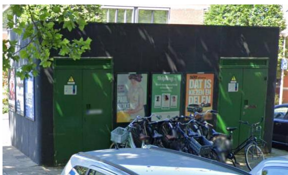
Figure 1-2 Current rectifier station Osdorp (front side)
