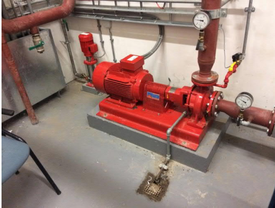
Sprinkler pump building T (Tias)
