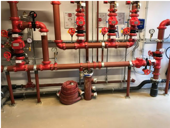
Alarm valves building Cube
