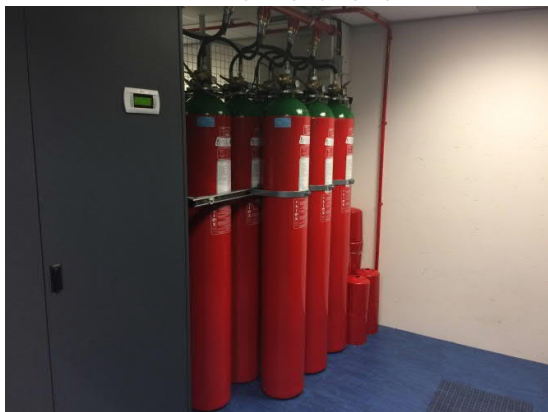
Argonite gas extinguishing system building S
