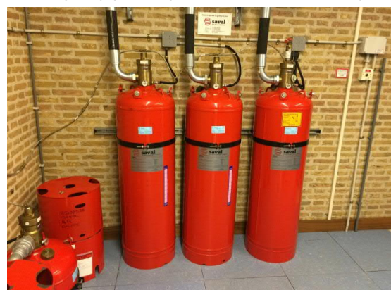
FM-200 gas extinguishing system building G
