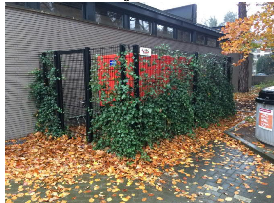
Emergency power generator next to building S
