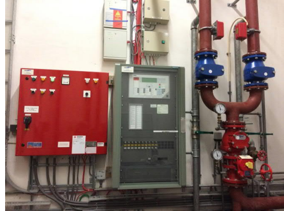
Sprinkler valves building T
