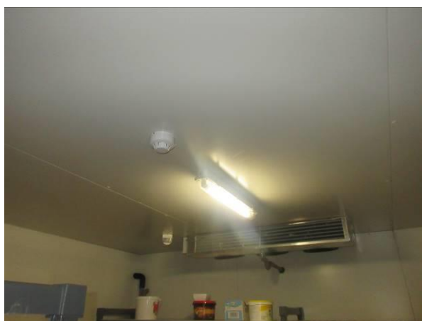
Rookmelder in koelcel
