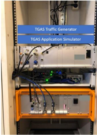
Figure 6 Free slots in the 19" rack of the MP Jules measurement train
