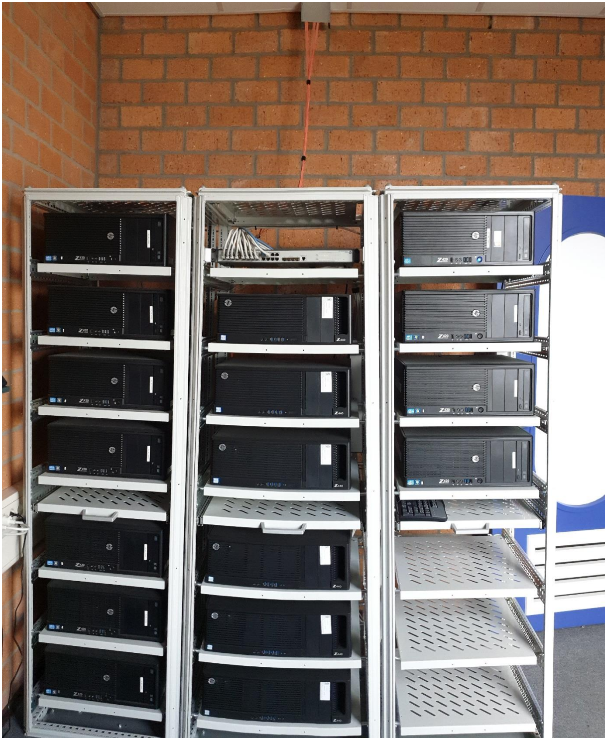
Computer racks with server, visual computers and network switch ( visual computers connected to monitors by fiberglass)
