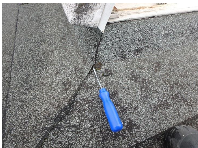
Foto 5 Onthechting overlap opstandstrook dakluik
